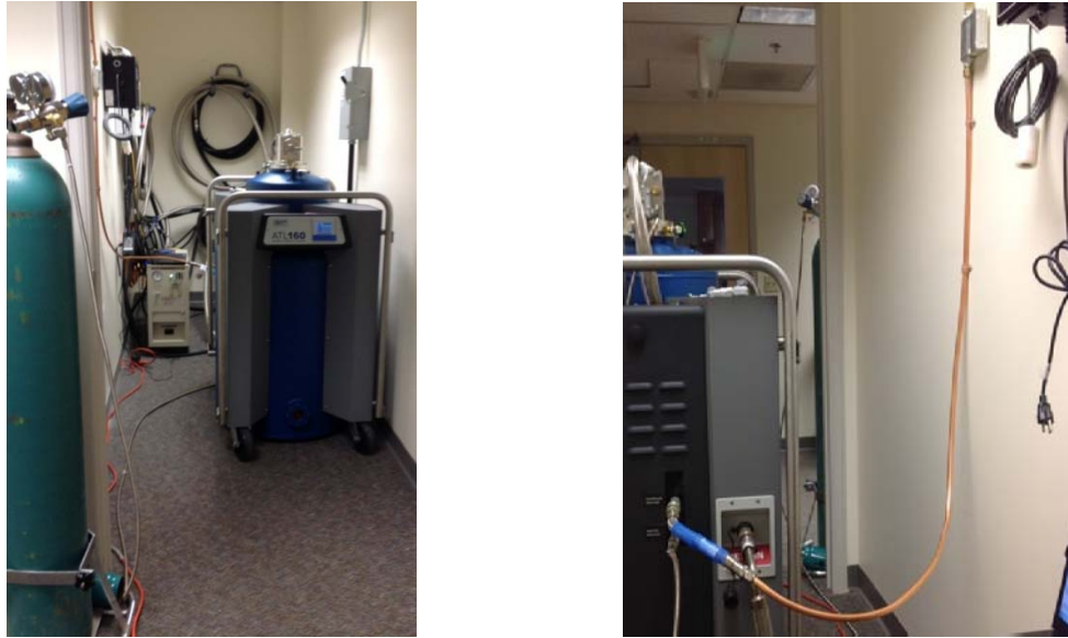
Figure 3 (left) ATL160 in the closet (right) Copper recovery line running to ATL160
